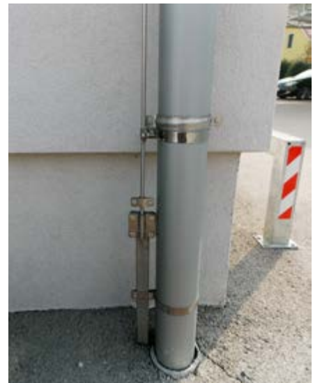
Figure 17: Downconductor, installed on the drain pipe
