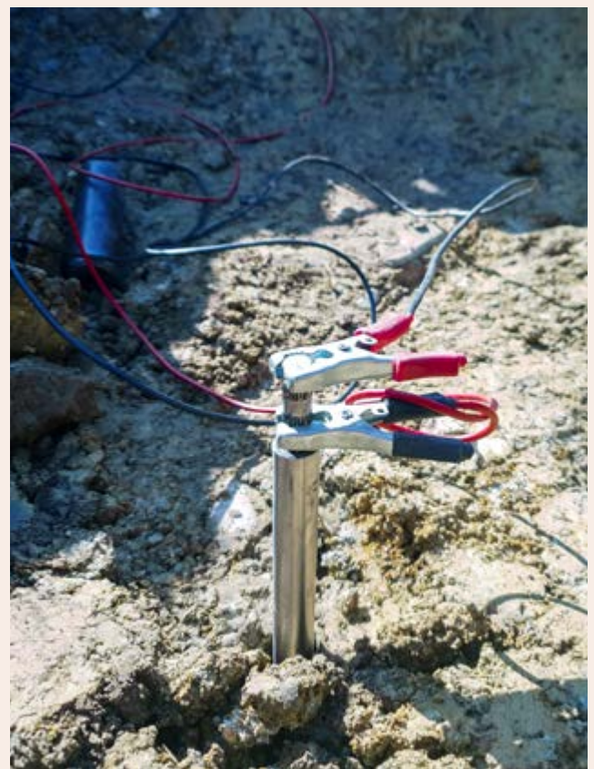
Figure 21: Example of an earthing device with a POS K Rf earth rod
