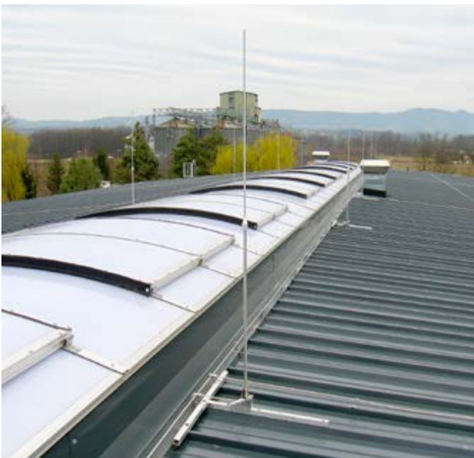
Figure 14: Catching rod mounted on the roof covered with trapezoidal tin sheet roofing
