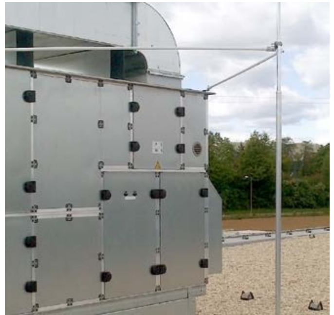
Figure 13: Catching rod mounted on a flat roof and additionally attached to the protected device by means of spacer elements.
