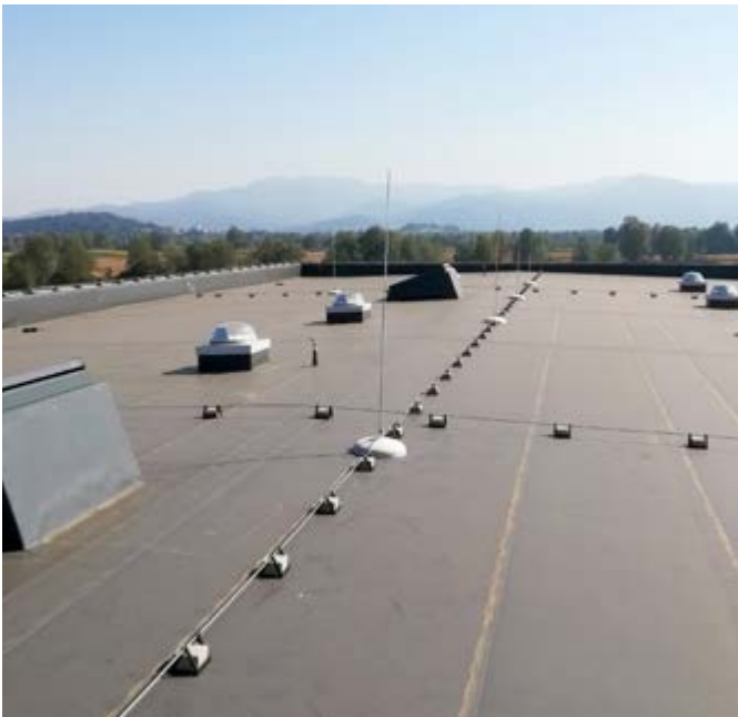
Figure 12: Catching rod mounted on a flat roof
