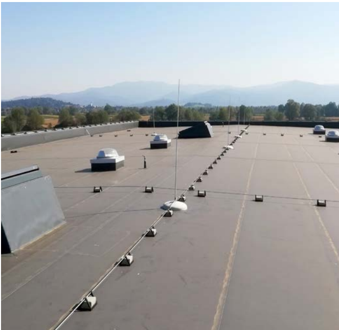
Figure 11: Catching rod mounted on a flat roof
