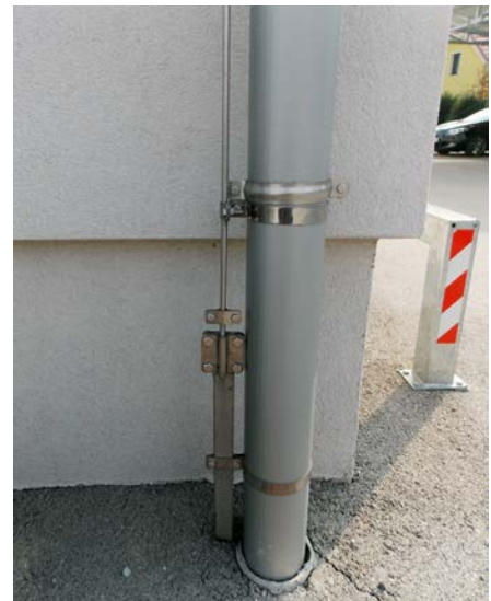
Figure 16: Downconductor, installed on the drain pipe
