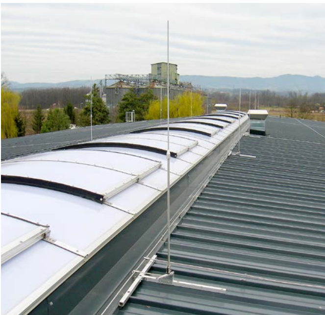
Figure 13: Catching rod mounted on the roof covered with trapezoidal tin sheet roofing
