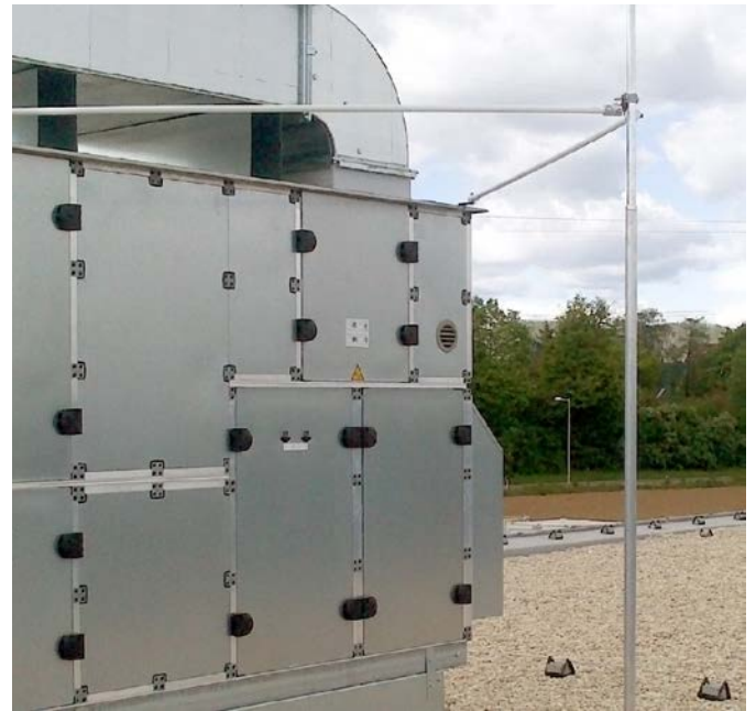
Figure 12: Catching rod mounted on a flat roof and additionally attached to the protected device by means of spacer elements.
